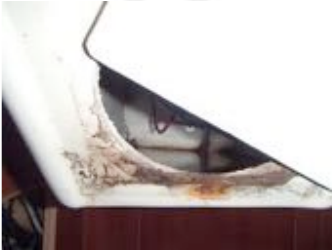
Image of a inspection panel removed on the underside of the starboard binnacle accessible form the starboard aft cabin. Note the water pooling at the base of this moulding.
