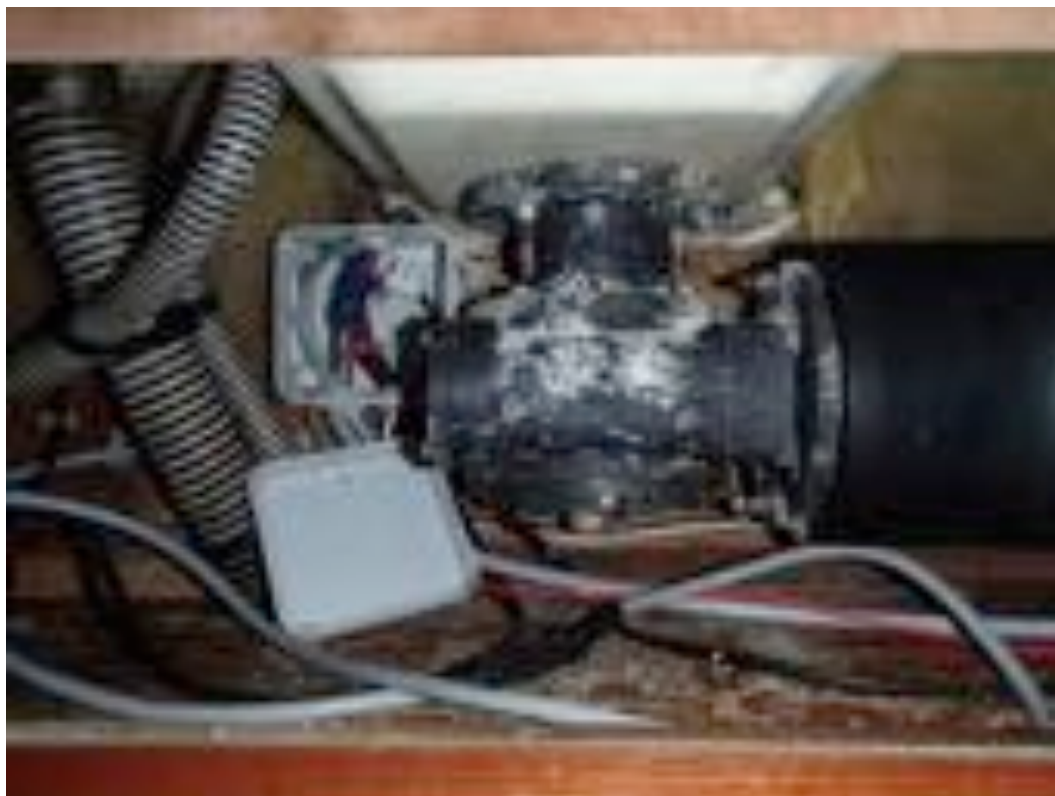
Image of the windlass motor from in a cupboard at the front of the forward cabin. Note the corrosion over the motor evidencing water ingress.
