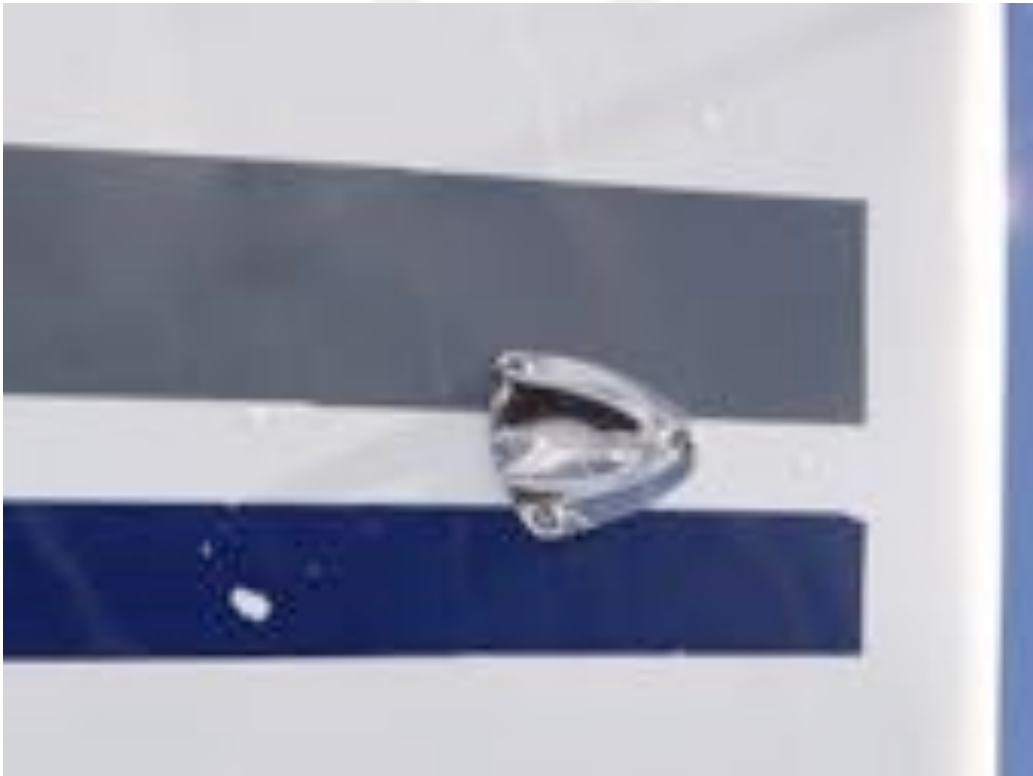
Image of the starboard chain locker drain deflector, noted deformed.
