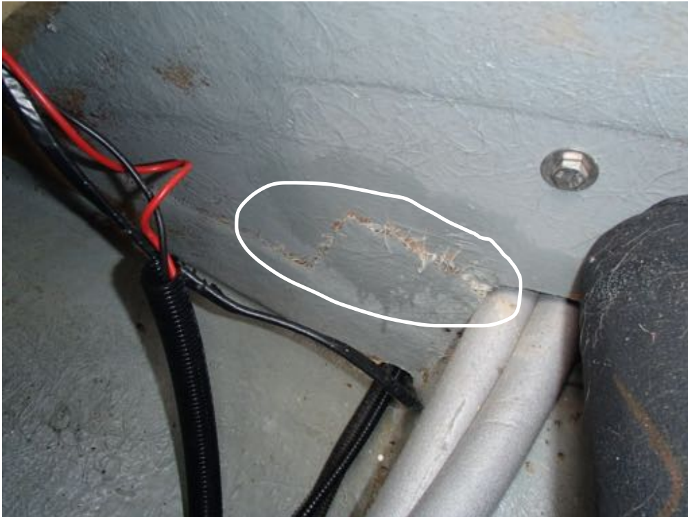
Image of a small section of the secondary bonding that has let go just forward of the fuel tank.
