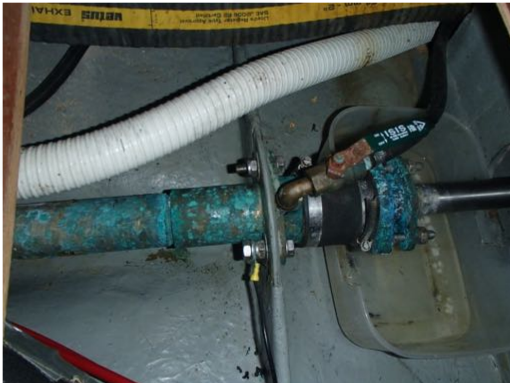
Image of the shaft seal. Note the surface corrosion and the container under the seal suggesting a leak.
