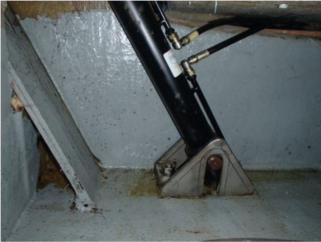
Image of the base of the swing keel hydraulic ram. An oil leak was noted.
