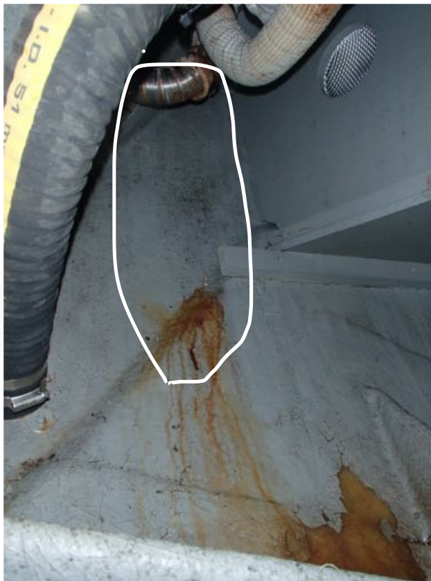
Image of a suspected leak from the heater exhaust or exhaust skin fitting
