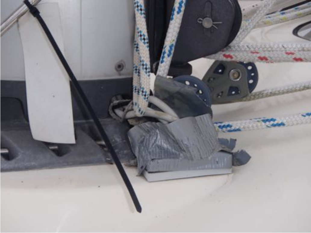
Image of the mast electric deck gland noted over taped
