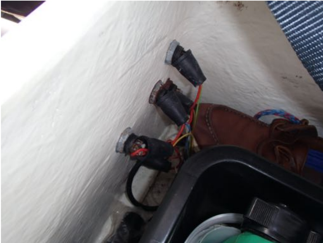
Image of the exposed and corroded switches for the passerelle.
