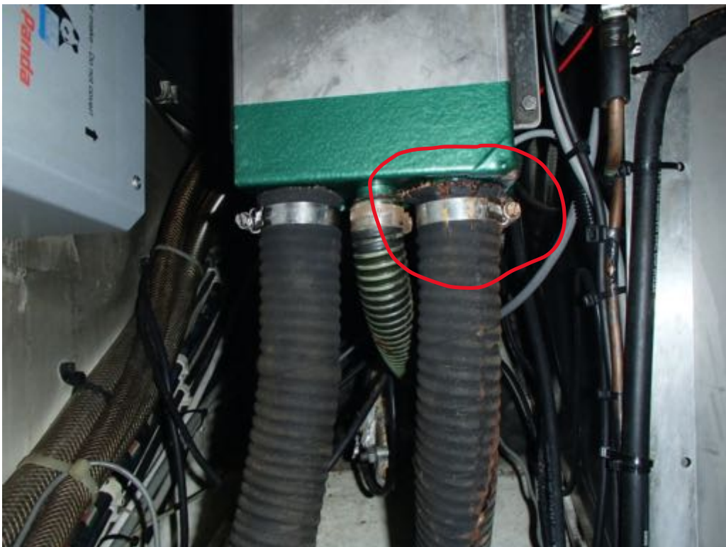
Image of the exhaust separator for the generator. A leak was noted.
