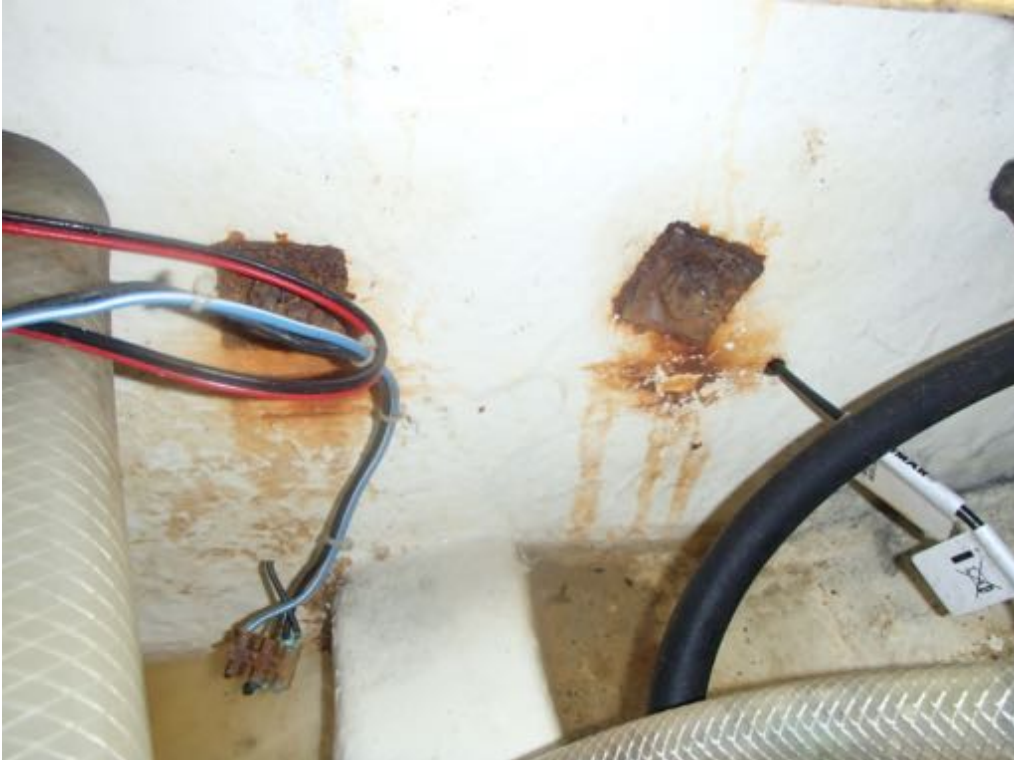
Image of the corroded bolts on the aft face of the bulkhead for the engine bearers.
